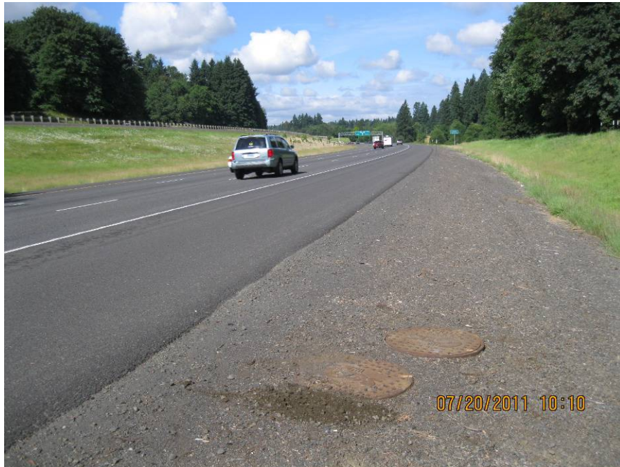
Photo 1: Looking west at WQ Manhole (CDS Unit).
