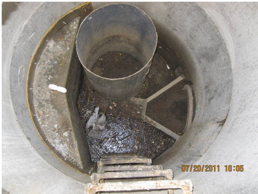
Photo 2: Inside view of WQ Manhole (CDS Unit).
