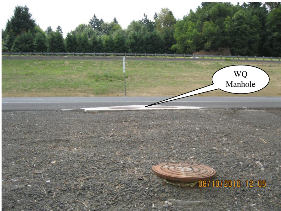
Photo 2: Similar to Photo 1 with a view of both the southbound (foreground) and northbound (background) travel lanes.
