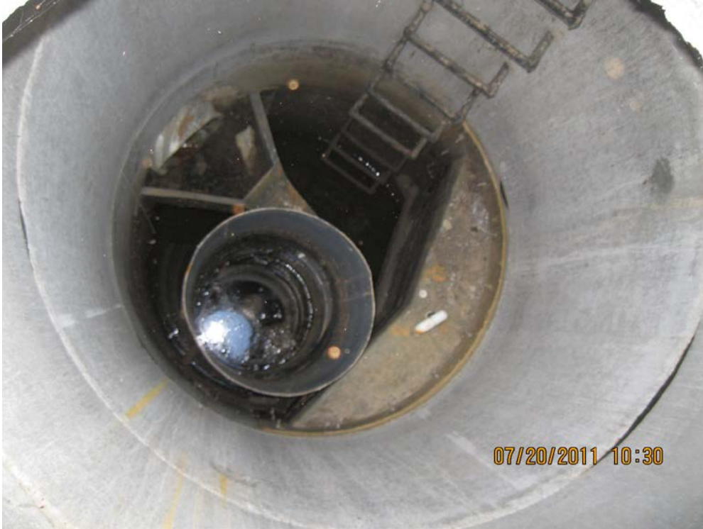
Photo 3: Inside view of WQ Manhole (CDS Unit).
