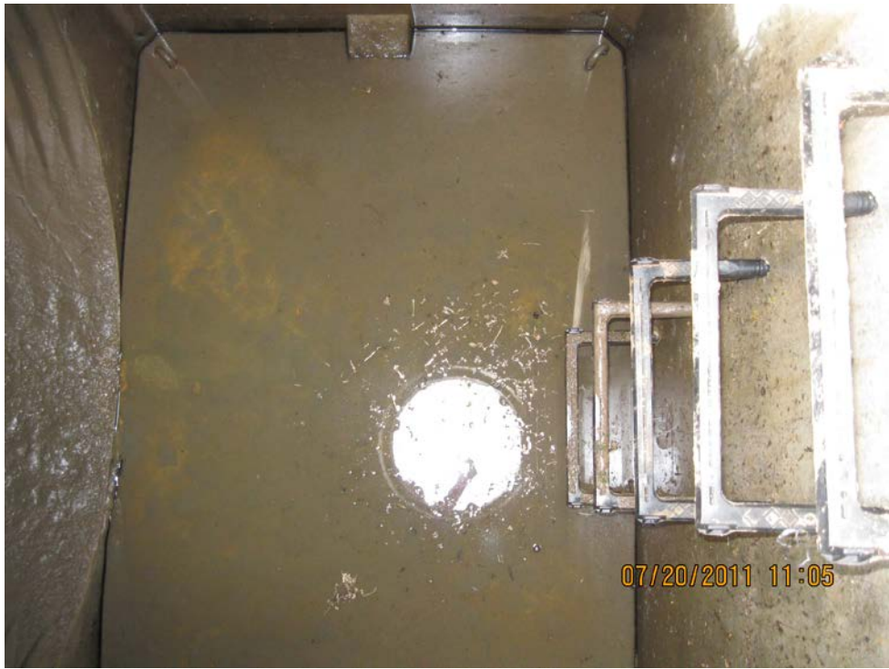
Photo 3: Looking down into inlet access vault (Point D).
