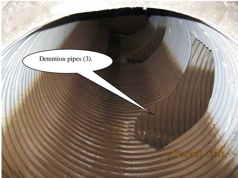
Photo 5: Looking at connecting manifold pipe from inlet access vault (Point D).
