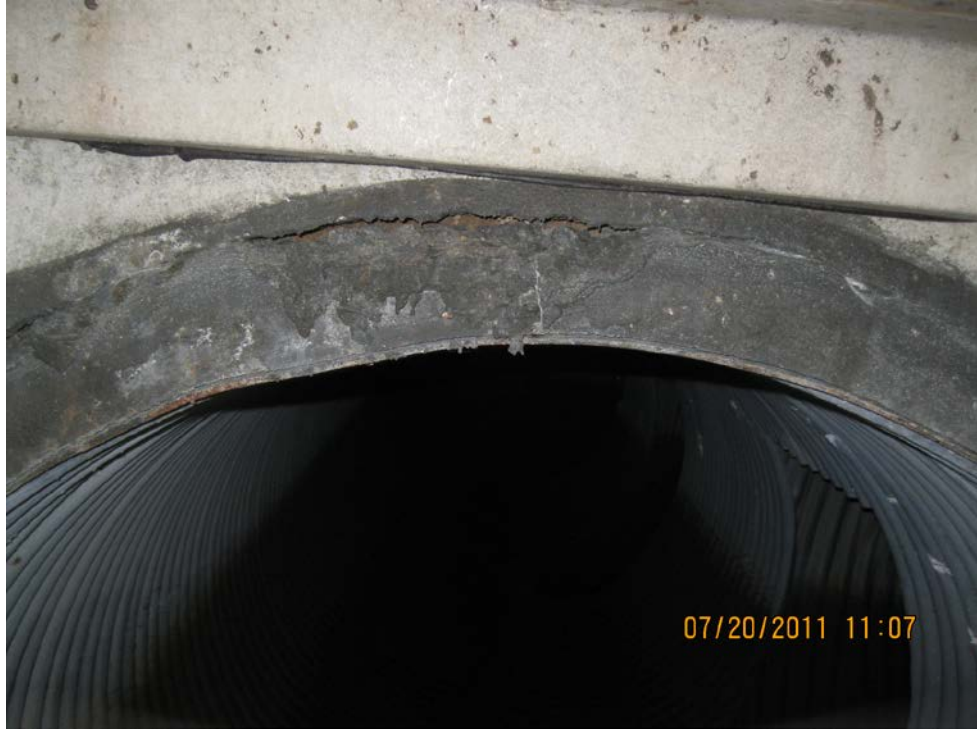
Photo 4: Looking at connecting manifold pipe from inlet access vault (Point D). Minor delamination is occurring in overhead header section of pipe.
