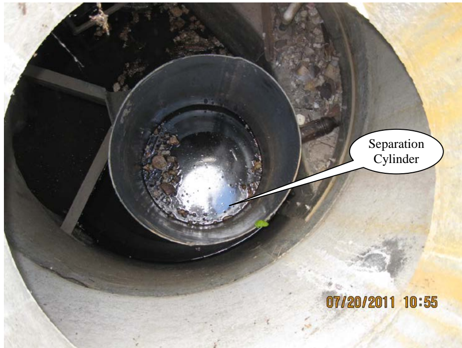
Photo 2: Internal view of water quality manhole (CDS Unit)
