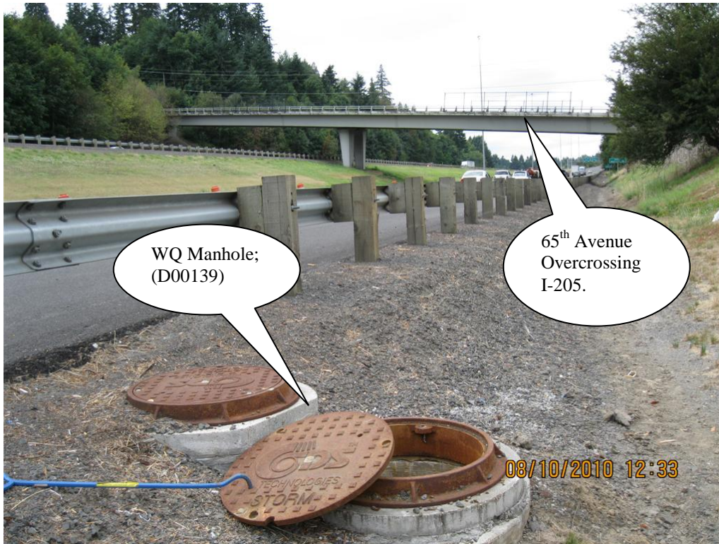
Photo 1: Looking west at the WQ manhole (CDS Unit); 65th Street overcrossing is in the background.
