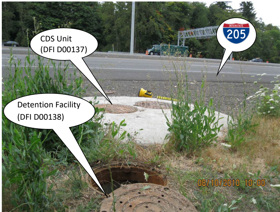
Photo 2: Rim of the inlet vault structure located on the northwest edge of the facility. WQ Treatment manhole, CDS Unit DFI D00137 located in the background (looking north).
