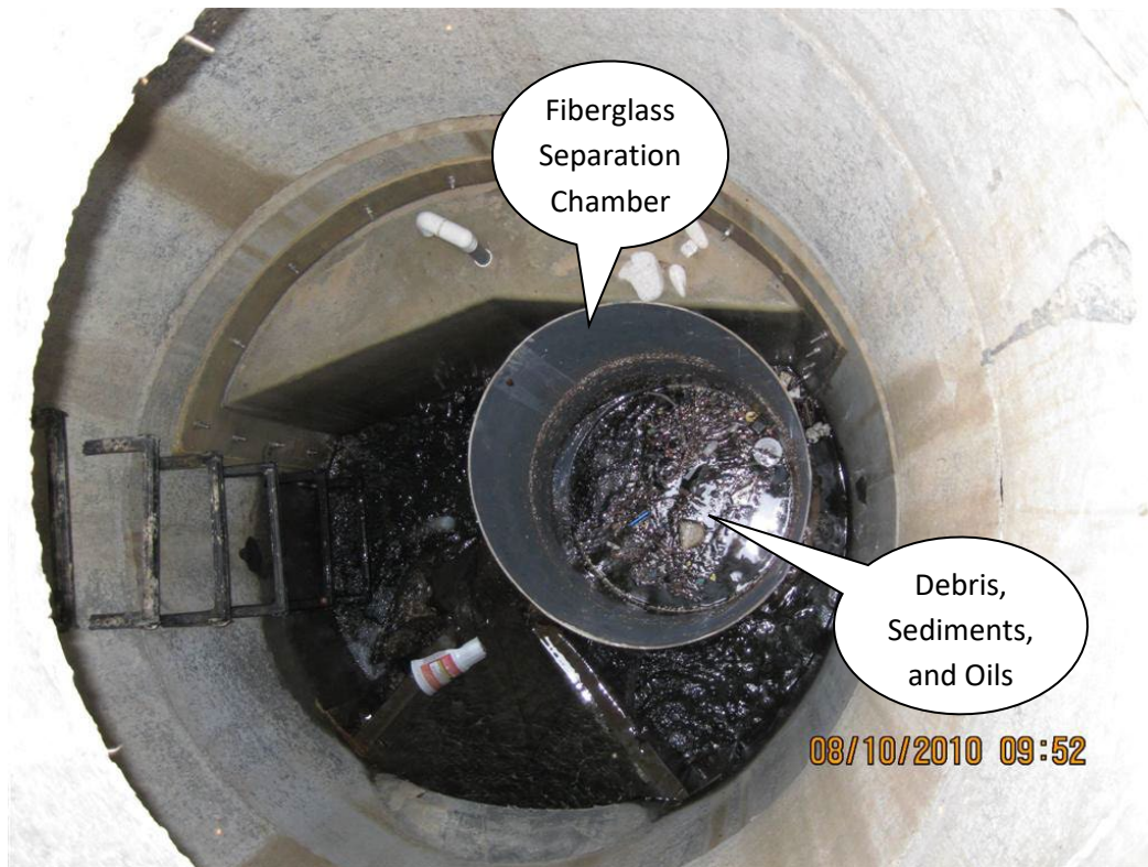
Photo 3: CDS Unit looking into from Rim. Facility Haz Mat Spill Feature(s)
