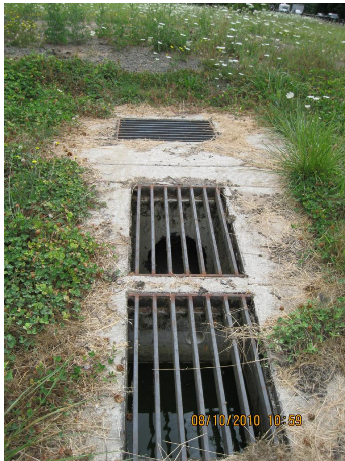
Photo 3: Lower and upper sections of the outlet control structure, showing 3-inch orifice and outlet pipe.
