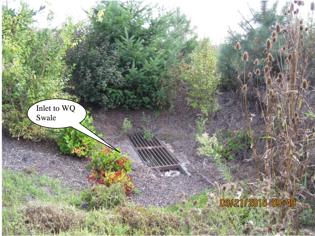
Photo 1: Modified Inlet acts, serving as an inlet to the WQ biofiltration swale; see Point C of the Operational Plan.
