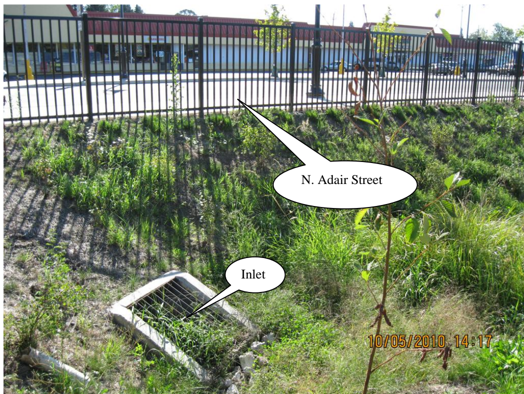
Photo 2: A look at the swale inlet located on the eastside of the facility
