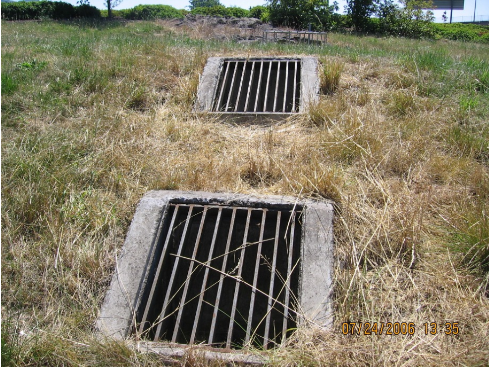
Photo 1: Overflow control structure looking south.
