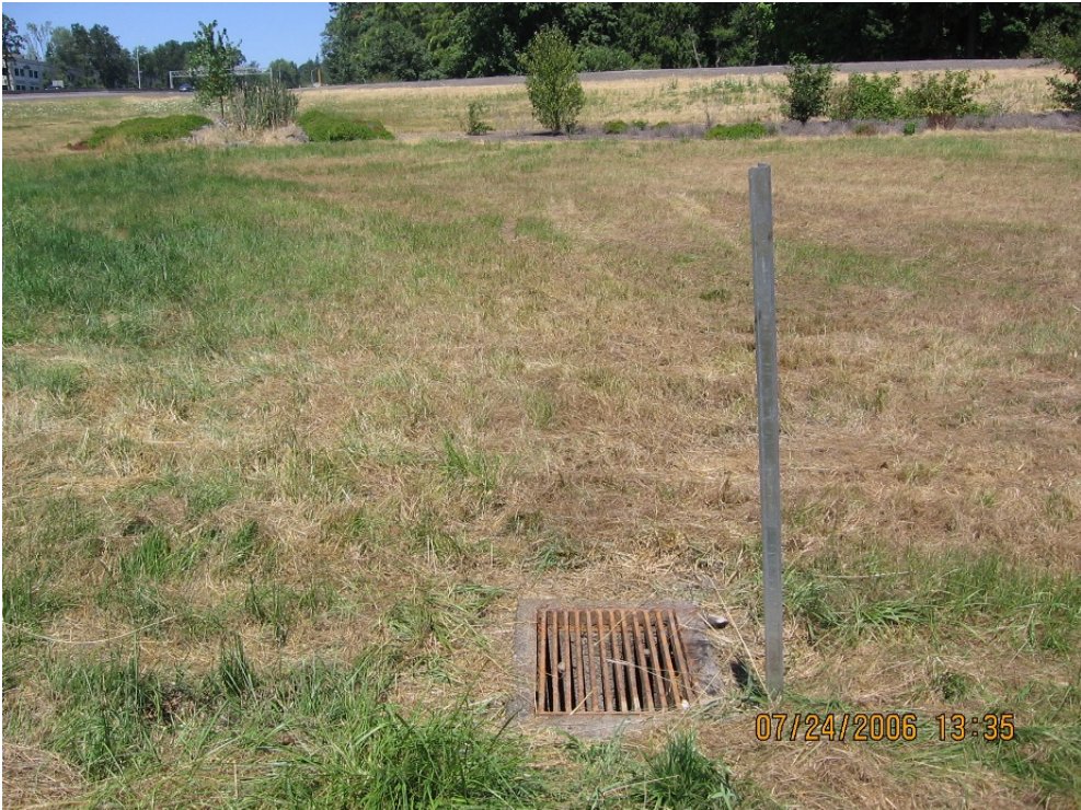
Photo 4: Old inlet within WQ Extended Dry Detention Pond that has been plugged. Inlet is no longer functioning.
