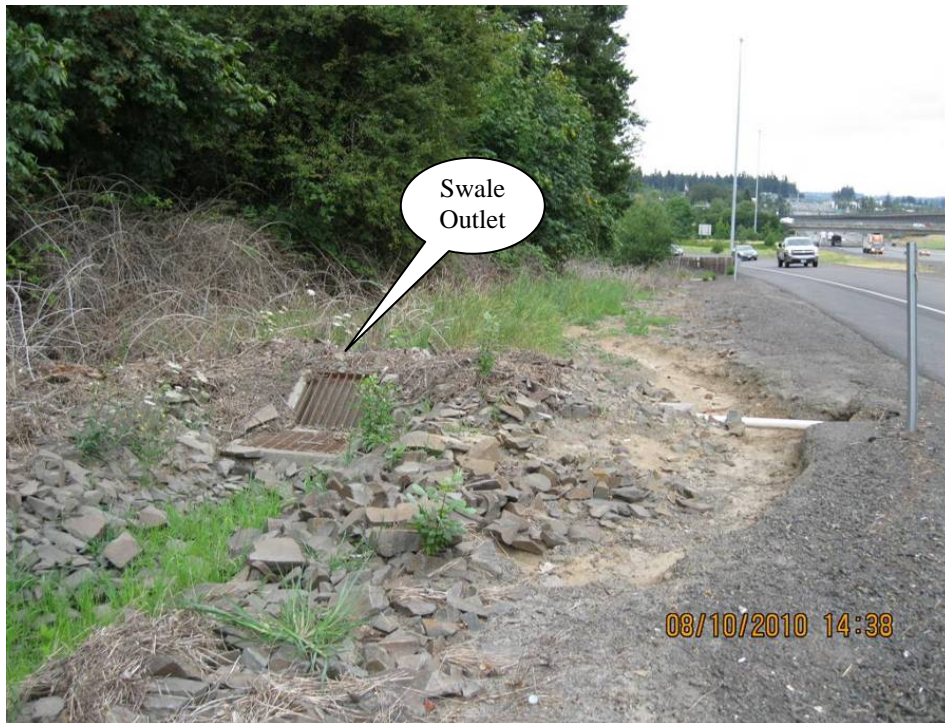
Photo 3: Swale outlet structure composed of two inlets. Flow from this structure is conveyed to WQ Facility DFI D00122 by a 36-inch storm pipe. There is evidence of the flow bypassing the outlet to the right.
