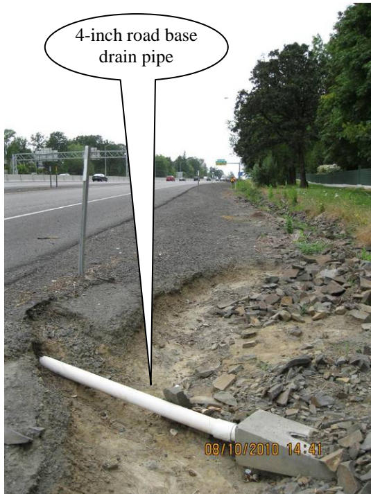
Photo 2: Road base 4-inch drain pipe outfall. There is evidence of highly erosive flow undercutting outfall's integrity.
