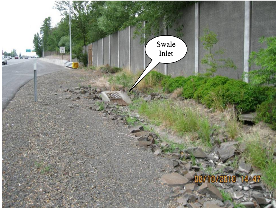
Photo 4: Swale inlet structure at the north end of the swale.
