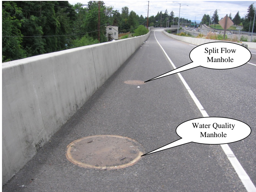
Photo 5: On-ramp from SW Canyon Road to eastbound lanes of US26 (Hwy 047.) Looking west, the water quality manhole is shown in the foreground. The split flow manhole is seen in the background.
