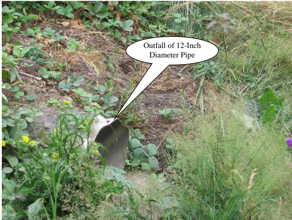
Photo 3: Outfall of 12-inch diameter pipe at swale inlet south of split flow manhole.
