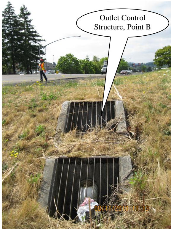
Photo 3: South outlet control structure, Point B, for the south treatment area.
