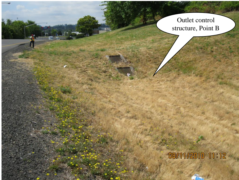
Photo 2: South outlet control structure, Point B, looking towards the south.
