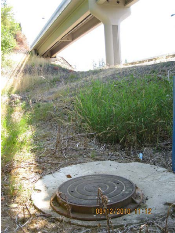
Photo 2: High-Low split flow manhole.
