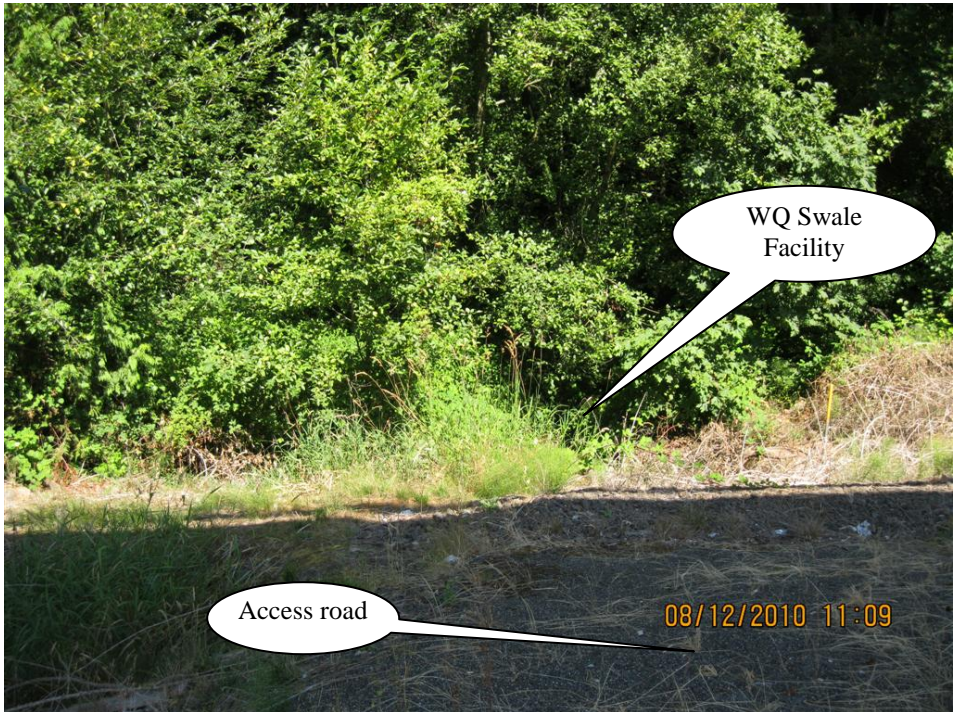
Photo 3: A photo of the water quality swale with significant vegetation and overgrowth.
