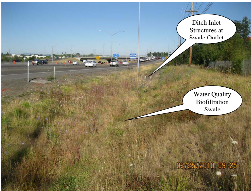
Photo 3: Location of ditch inlet structures at outlet of water quality biofiltration swale (DFI D00111.) Photo taken facing west.
