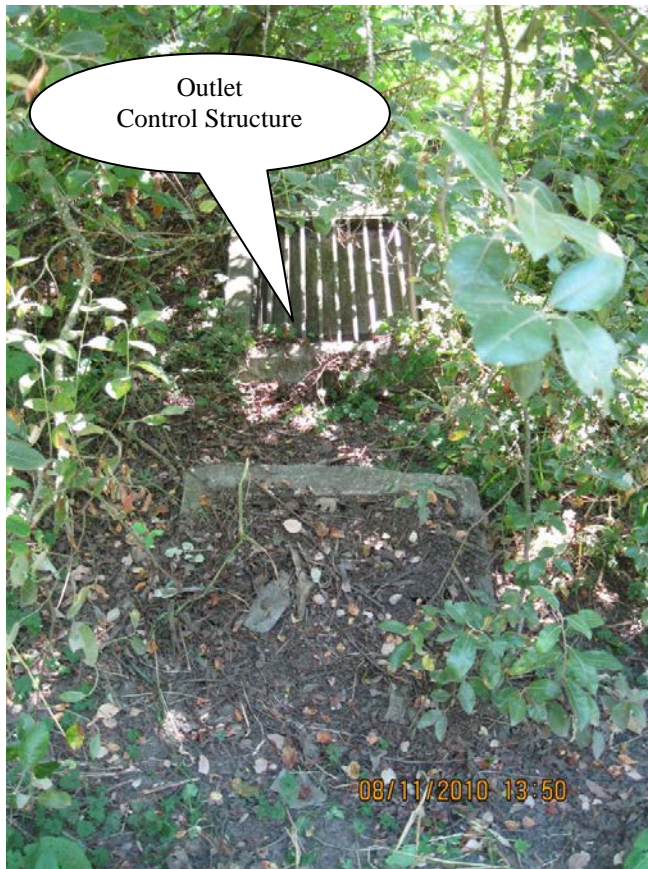
Photo 1: Outlet control structure for extended dry detention pond facility. Primary inlet appears plugged and is in need of maintenance.
