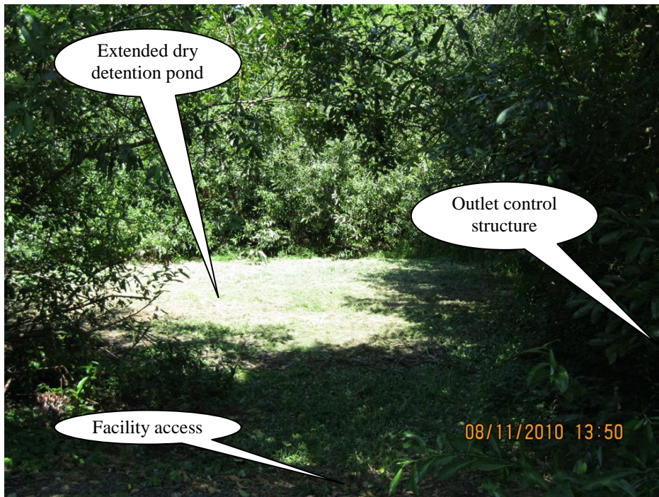
Photo 2: Extended dry detention pond. Vegetation surrounds the perimeter. Outlet structure is located to the right. Foreground shows the access from S.W. Benz Park Dr.
