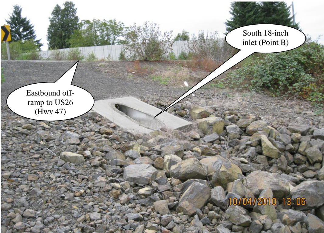
Photo 2: Detention pond facility at south 18-inch inlet (Point B). This inlet directs flow from the grassy swale of DFI D00129.
