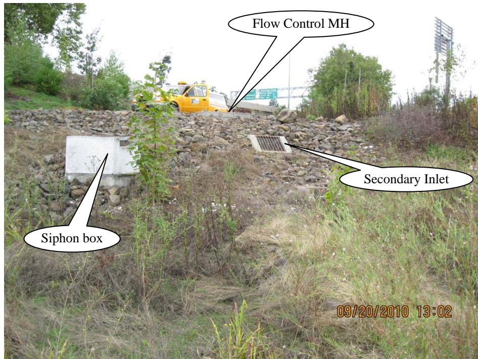
Photo 3: Outlet Control Structure including the high flow secondary ditch inlet, a flow control manhole and a siphon box to the left. All water entering the pond exits here.
