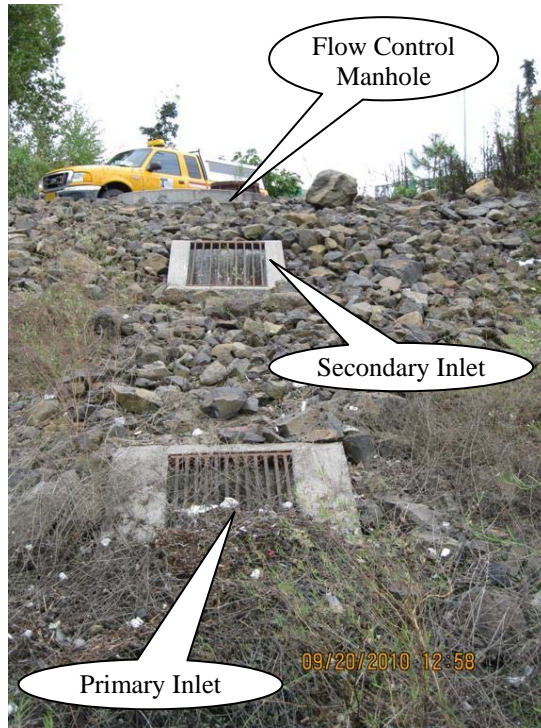
Photo 2: Outlet Control Structure comprised of both a primary and secondary set of ditch inlets, acting as the facility outlet with the flow control manhole in the background. All water entering the pond exits here.
