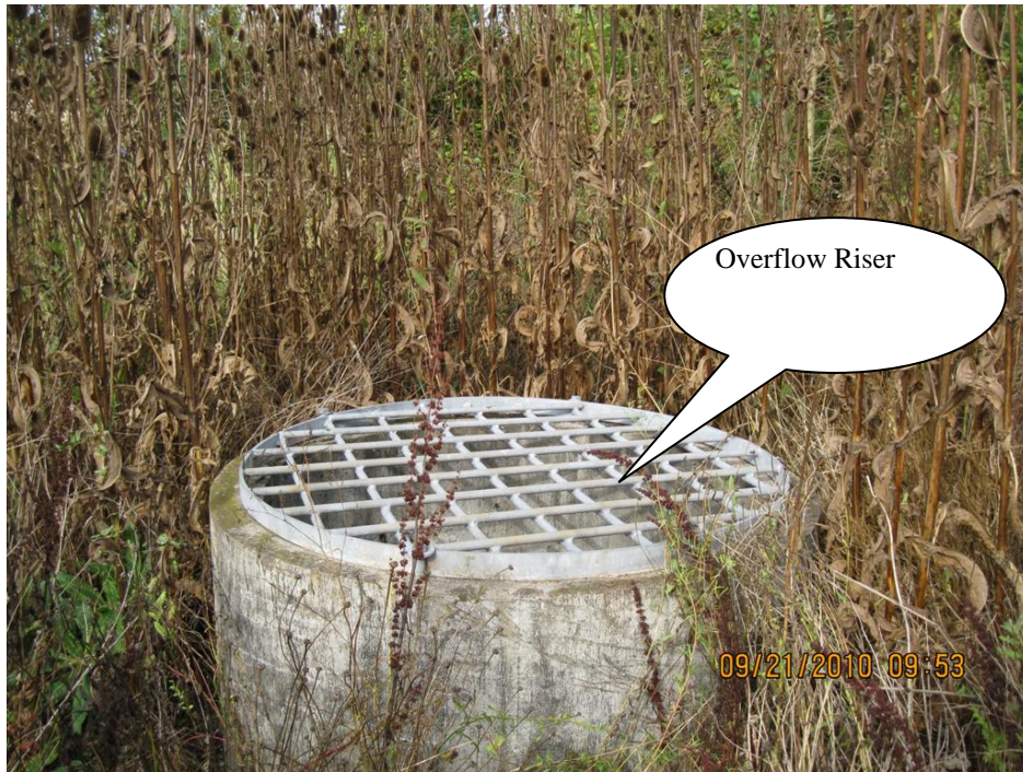
Photo 3: Overflow riser manhole for extended detention dry pond, (Point D, Operational Plan)
