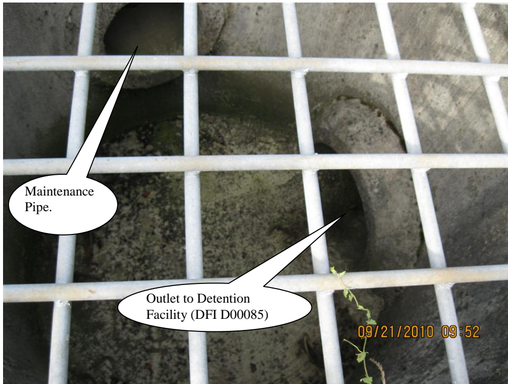
Photo 4: Overflow riser manhole from rim. Inlet at the top of the picture is intended for maintenance purposes and otherwise commonly plugged at all times, (Point D, Operational Plan)
