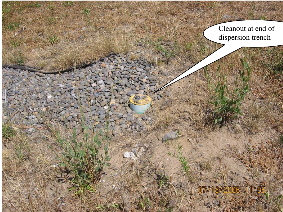
Photo 4: Typical cleanout for dispersion trench.
