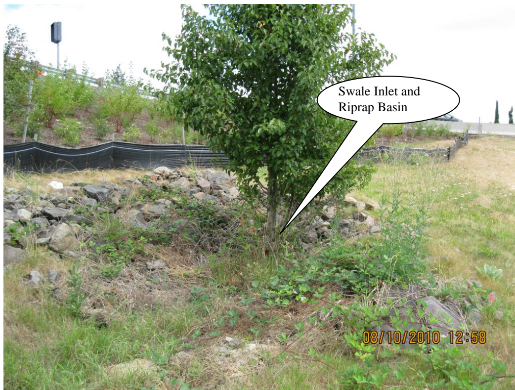
Photo 7: Swale Inlet and Riprap Basin. Tree located within basin poses potential problems including inhibiting the flow, breaking the outlet pipe, and causing erosion or possible failure of the nearby berm.
