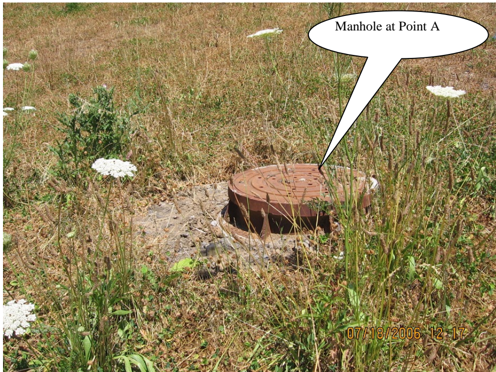
Photo 5: Manhole at Point A. Provides pretreatment by collection of sediments with sump.
