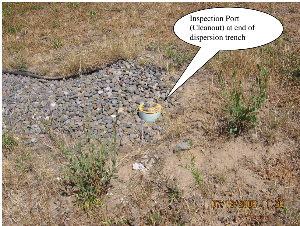
Photo 3: Typical inspection port (cleanout) for dispersion trench.
