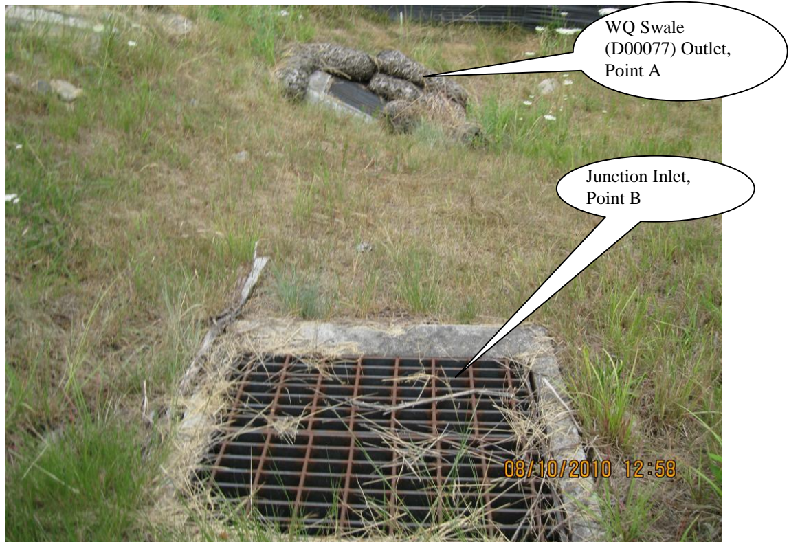
Photo 1: Junction Inlet (Point B) in the foreground. Swale outlet ditch inlet of D00077 in the background.
