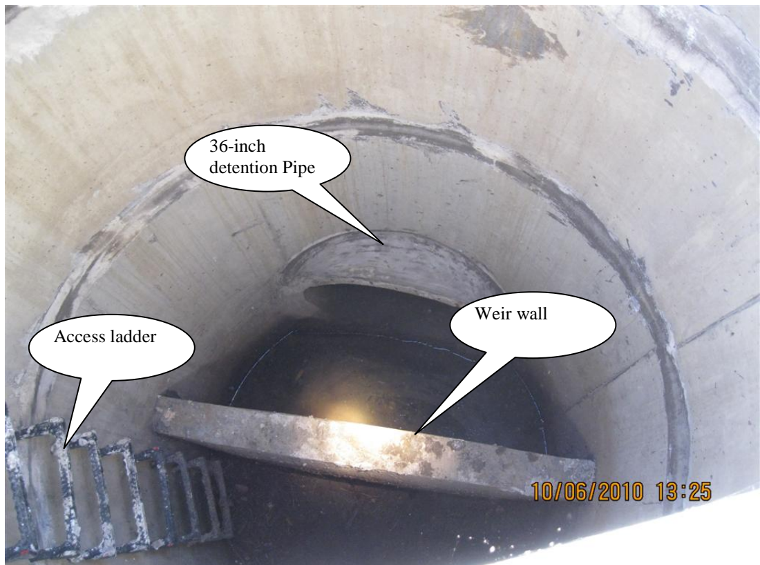
Photo 2: 72-inch diameter manhole (Point B) midway between two each 36-inch detention tank/pipes. This manhole contains a 4-foot high baffle.
