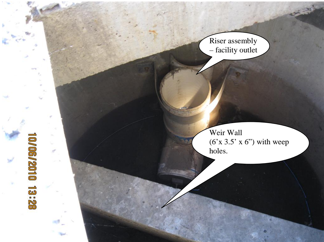
Photo 3: Outlet control structure (Point C) for 36-inch diameter detention tank/pipes. Flows exit system through riser pipe.
