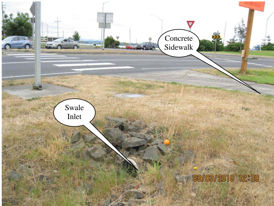
Photo 1: Swale Inlet, 12-inch culvert pipe, at the southern portion of the swale. A 10-foot wide concrete sidewalk is shown to the right.
