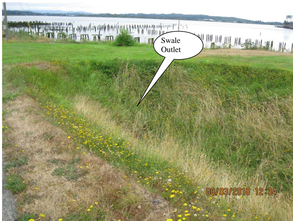
Photo 4: Swale outlet (Point B) and nearby manhole (Point C) looking south towards Young's Bay.
