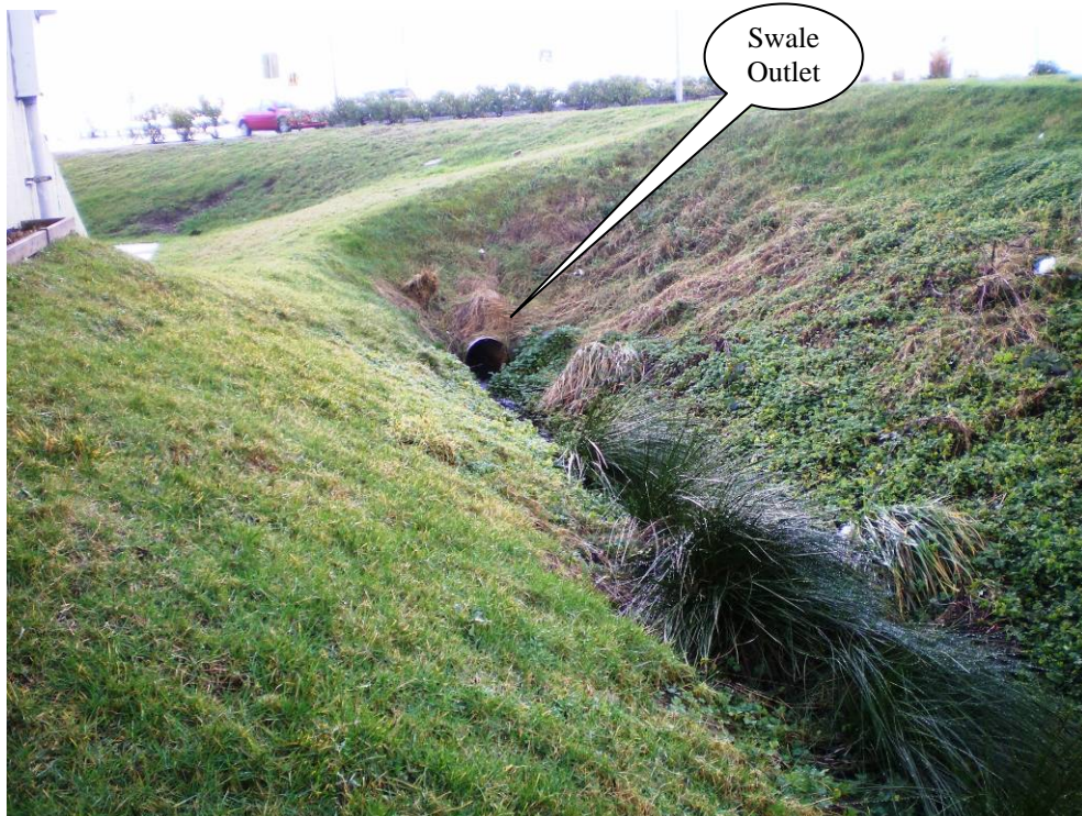
Photo 4: Photo looking south at swale outlet, 18-inch storm at corner of pump station.
