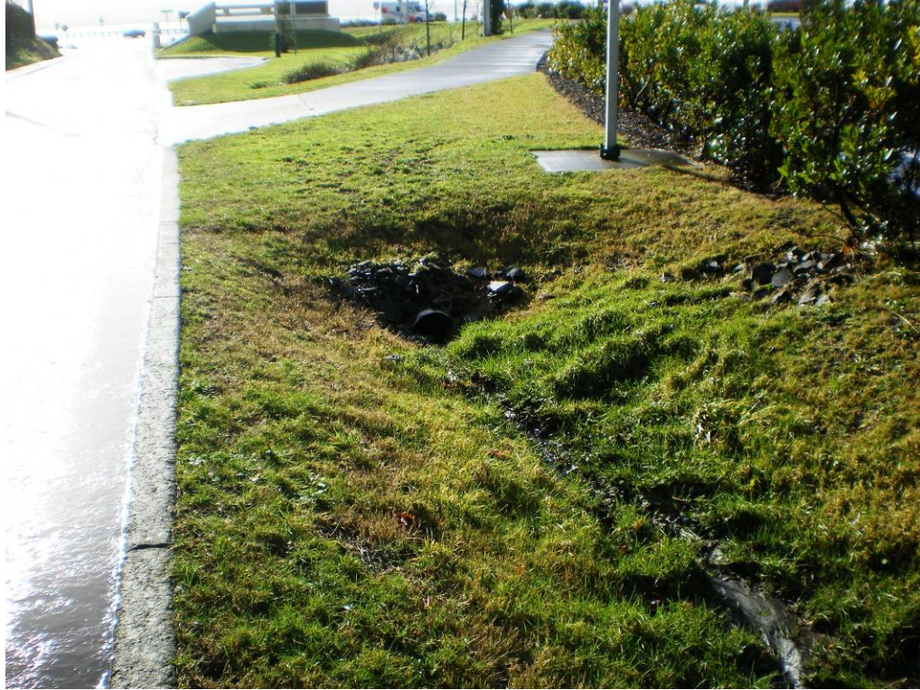
Photo 7: Swale Outlet, 12-inch culvert pipe, at the southern portion of the swale.
