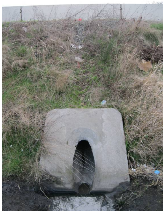
Photo 7: Northern central pipe outlet into swale (Point E on Operational Plan in Appendix A).
