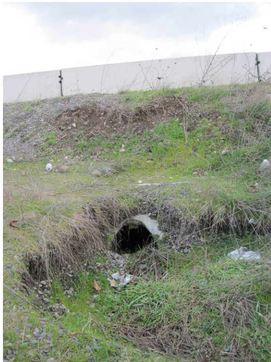
Photo 5: Southernmost pipe outlet into swale (Point C on Operational Plan in Appendix A).
