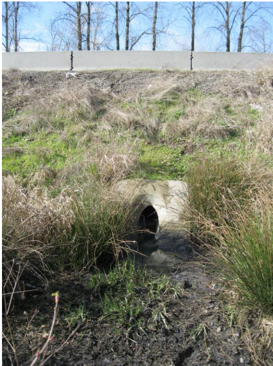
Photo 4: Southern conveyance pipe outlet (Point D on Operational Plan in Appendix A).
