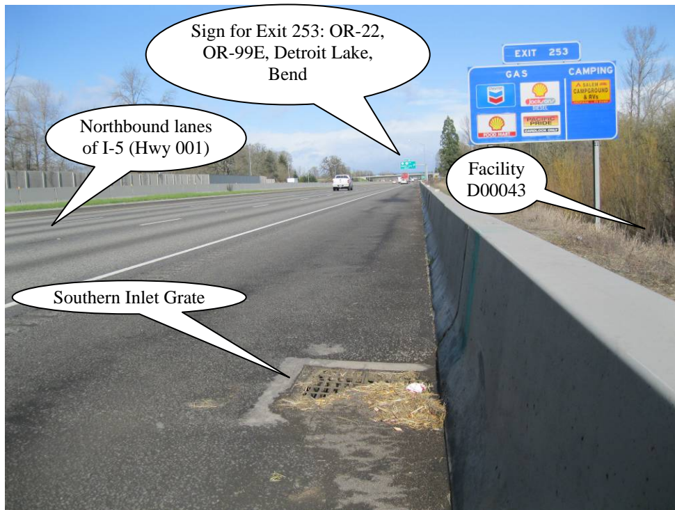
Photo 3: Facility D00043 receives stormwater from the adjacent southbound and northbound lanes of I-5 (Hwy 001).
