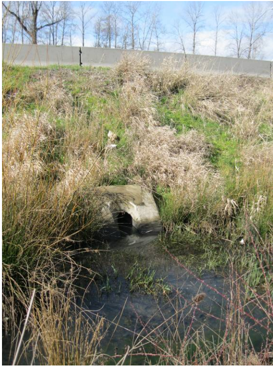
Photo 5: Northern conveyance pipe outlet (Point E on Operational Plan in Appendix A).
