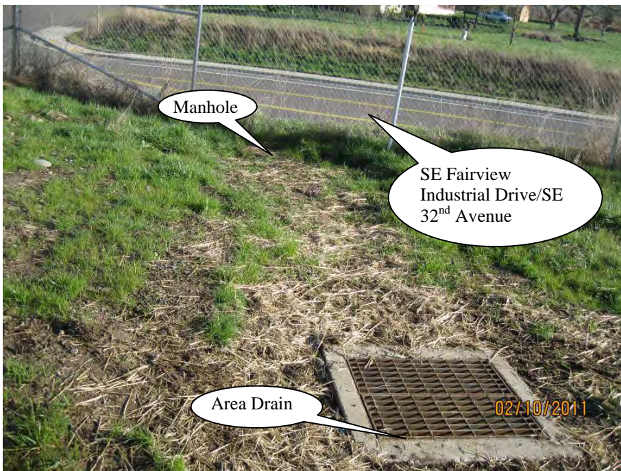
Photo 10: Manhole at connection between facility conveyance line and pipe from area drain in the foreground (Point F on the Operational Plan in Appendix A). The facility conveyance line discharges into the stormwater system underneath SE Fairview Industrial Drive/SE 32 nd Avenue.
