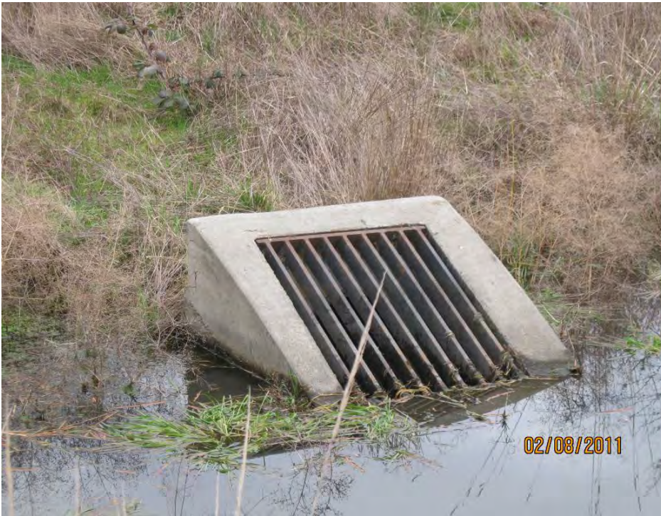
Photo 5: Ditch inlet structure at north end of pond/swale combo (Point D on the Operational Plan in Appendix A.)
