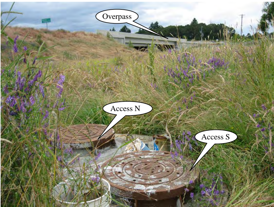
Photo 6: Photo looking north at the flow control manhole (two access lids) in the foreground and the SE Fairview Industrial Drive overpass in the background. (Point E on the Operational Plan in Appendix A.)
