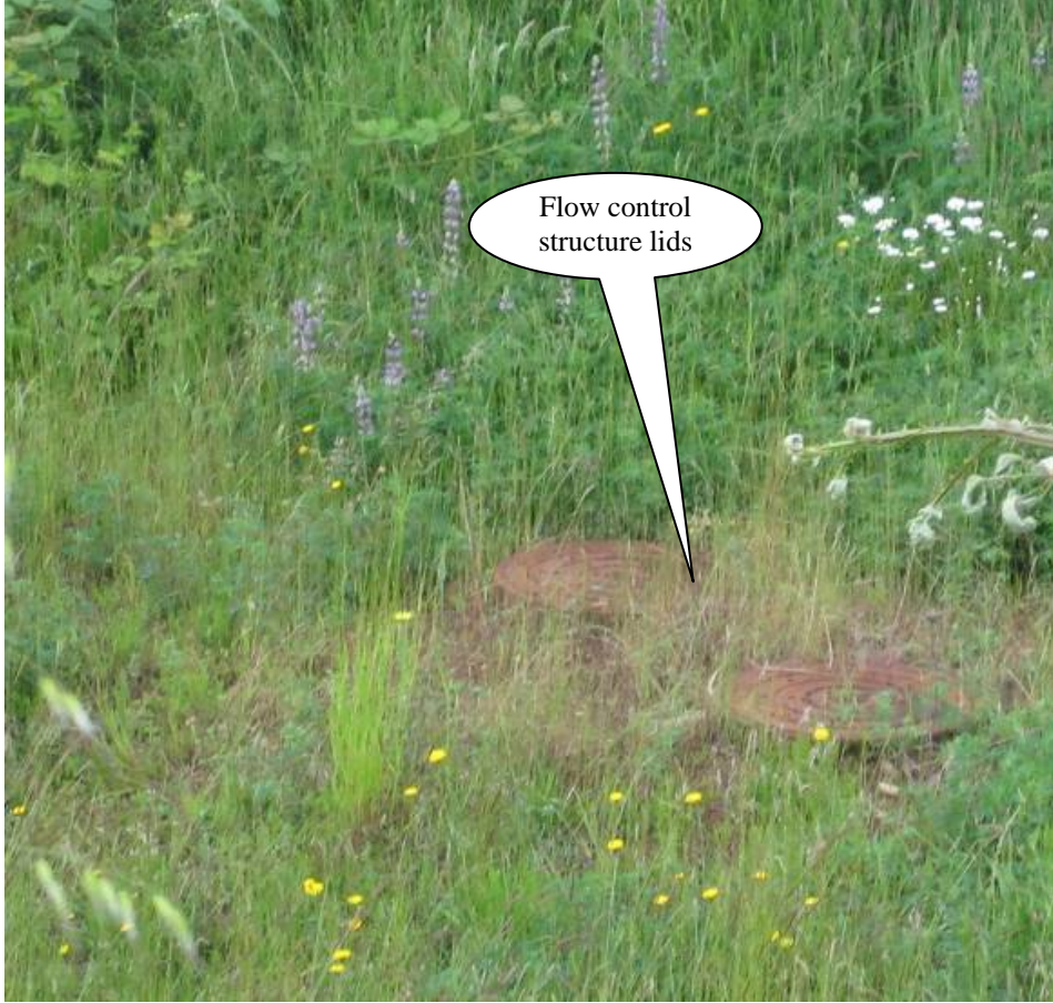
Photo 2: Flow control structure with double lids located in the northwest corner of the pond
