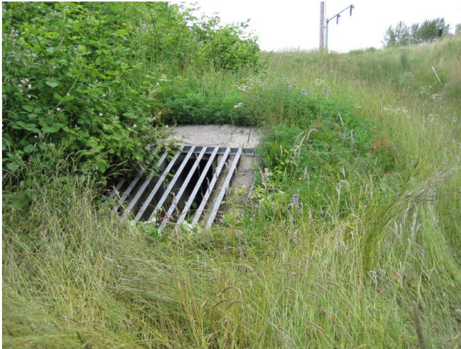
Photo 5: Look west at 27-inch storm drain pipe with metal grate (Point H on Operational Plan). This pipe drains into the flow control manhole.
