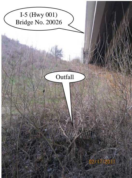
Photo 3: Outfall to ditch. This outfall discharges stormwater from D00038 as well as D00039 and D00034. The picture was taken facing south.
