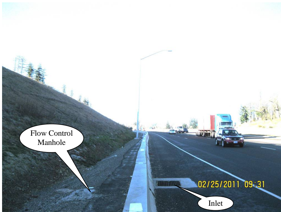
Photo 2: The facility drainage area is approximately 1,970 feet of the northbound lanes of I-5 (Hwy 001.)
