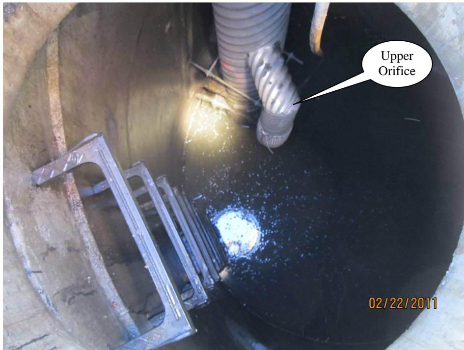
Photo 3: This photo is looking in the interior of the flow control manhole.
