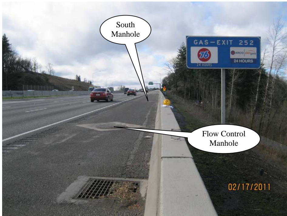
Photo 1: Detention pipe facility looking south. Detention pipe is located between the flow control manhole and the south manhole.
