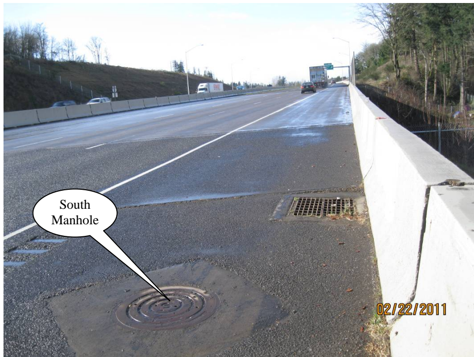
Photo 2: This photo is looking at the south manhole located on south end of detention facility.
