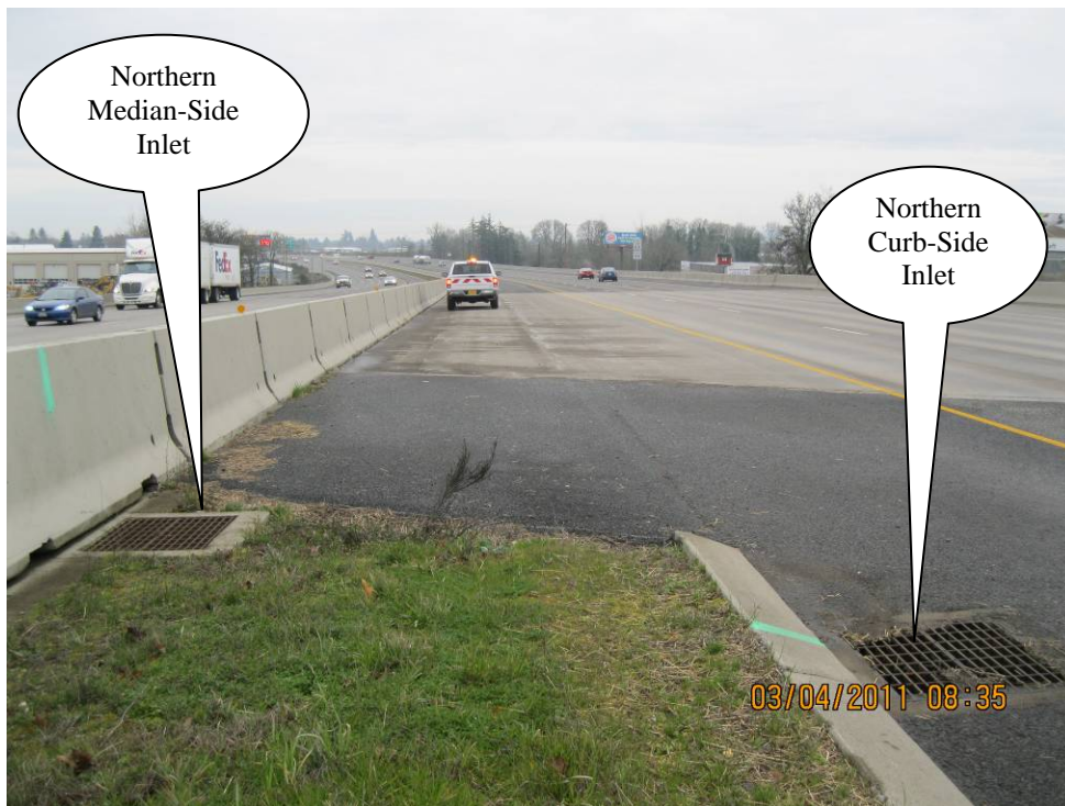
Photo 2: Northern inlets. The manhole between these inlets was not found during fieldwork, but construction photographs confirm that the manhole exists. For the position of this manhole, refer to the Operational Plan in Appendix A and pages 16C and 16D in 38V-117 in Appendix B.
