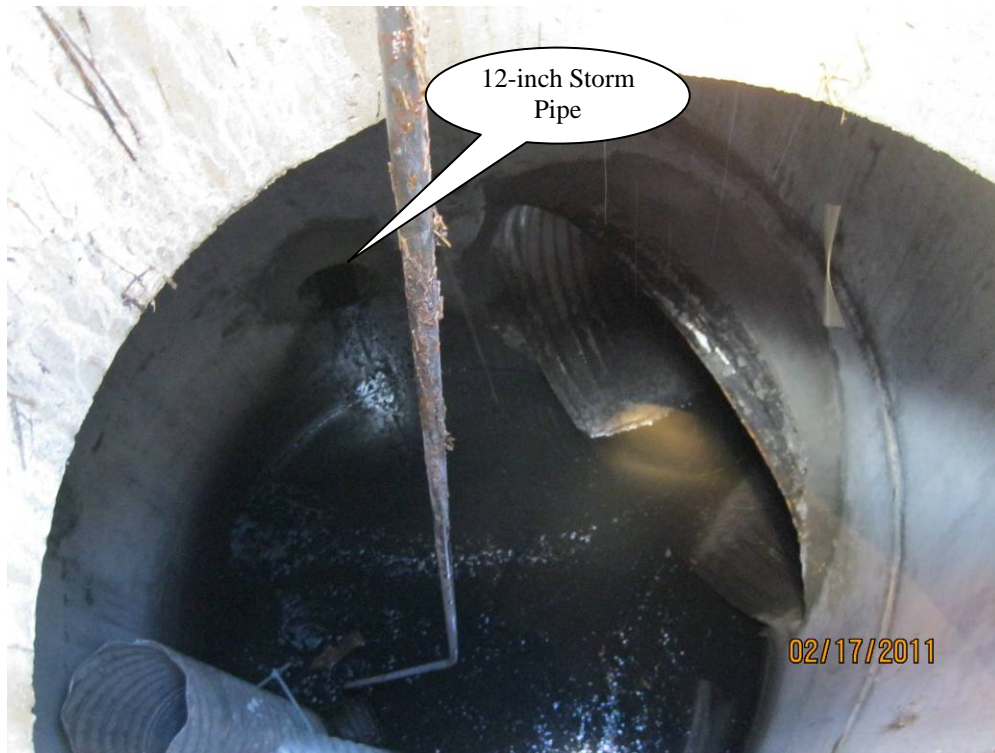
Photo 4: Interior of flow control manhole similar to Photo 3. This photo provides a view of the 12-inch storm inlet providing flow into the detention structure.
