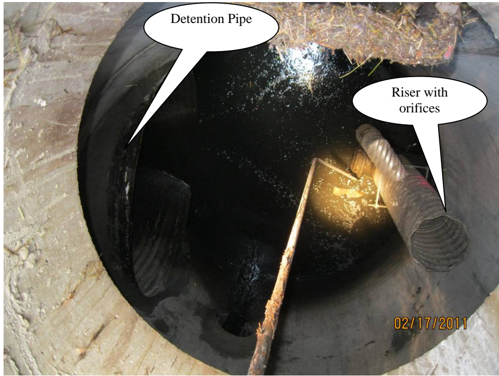
Photo 3: Interior of flow control manhole. Detention pipe is to the left. The riser and orifice structure located to the right. The rod in the middle of the structure connects to a valve that drains the structure in event the orifices are plugged.
