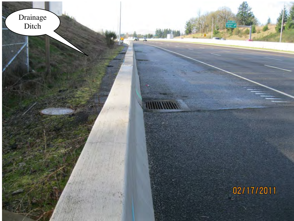
Photo 3: Area of highway that drains towards facility. To the left is the roadside ditch that is collected by the ditch inlet adjacent to the water quality manhole.
