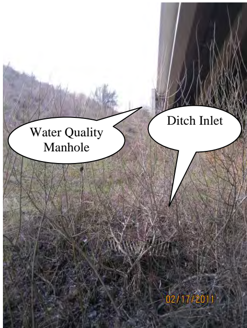
Photo 6: The ditch inlet (2 grates) serves as the outlet structure for the stormwater treated through the water quality manhole facility.
