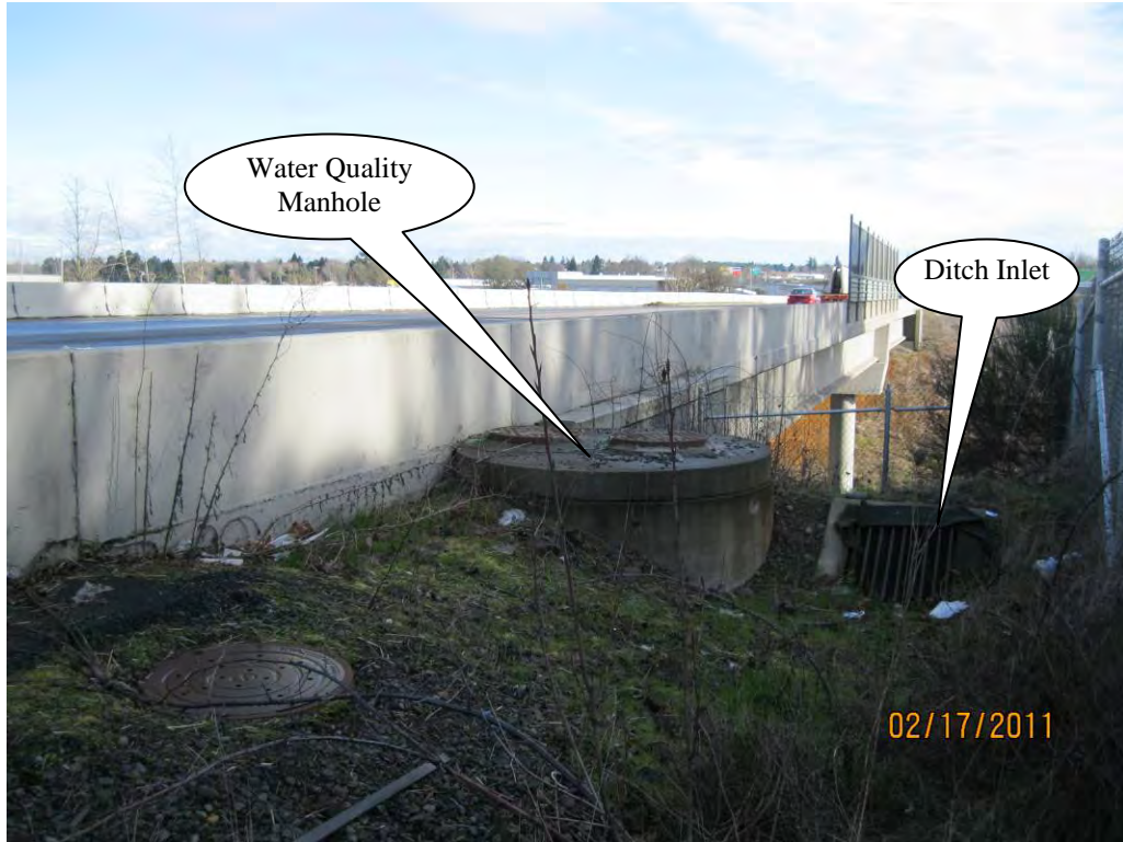
Photo 1: Photo looking at water quality manhole and ditch inlet towards the north at the U.P.R.R corridor overpass.
