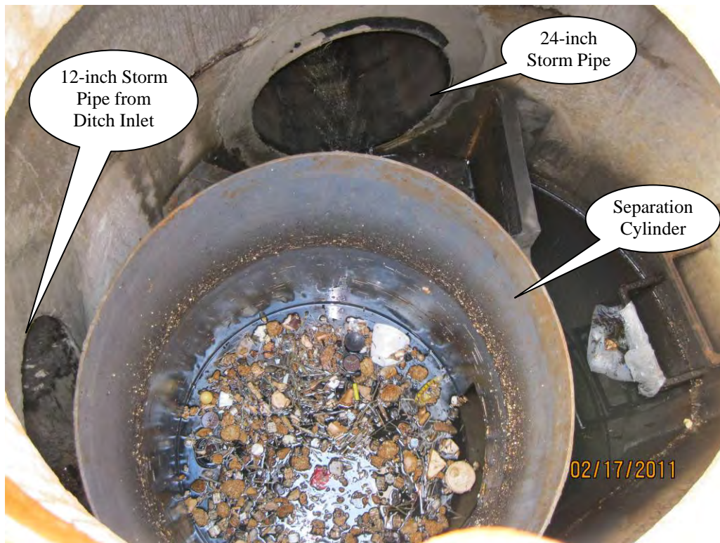
Photo 4: Inside view of water quality manhole looking at separation cylinder filled with floating debris.
