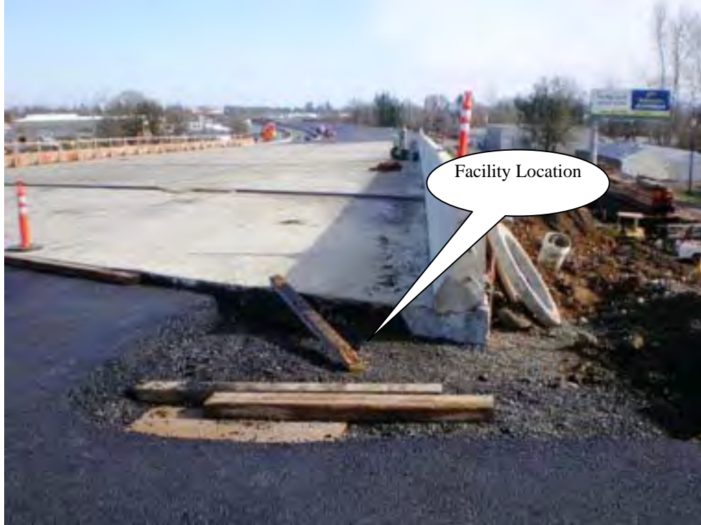
Photo 1: This photo depicts the location of the water quality manhole at the edge of the end panel of Bridge No. 20032.
