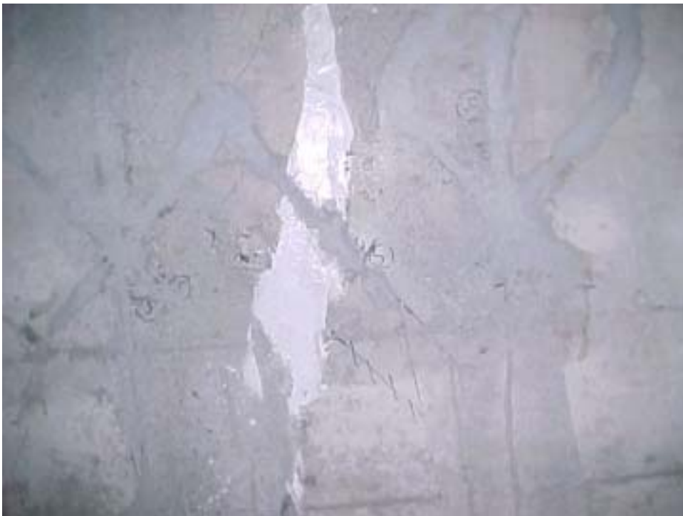
Figure B.3: Appearance of sensor locations after the grooves were filled with grout
