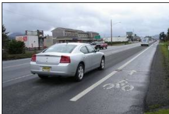
Figure 2.5: US 101 Bicycle Lane with Gravel and Debris Stretching Down the Middle of the Lane
