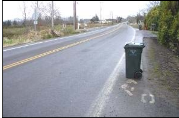
Figure 11: Narrow Bike Lane on Lewis and Clark Road with Trash Can Blocking Lane
