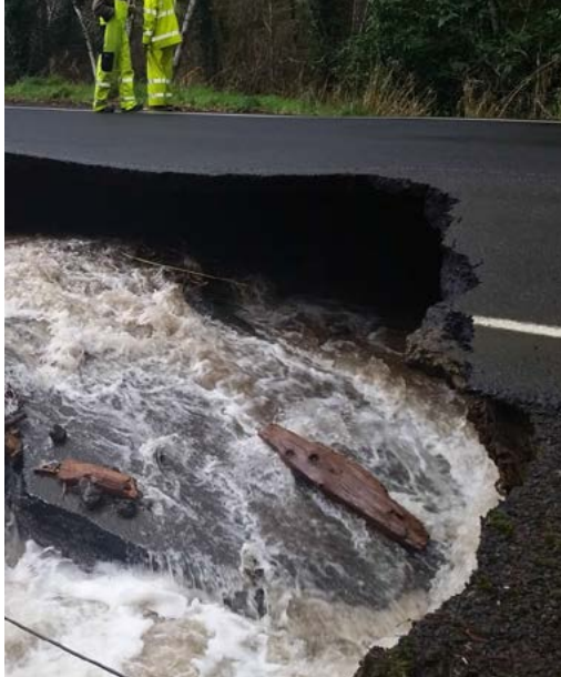
When culverts failed, inundation and debris did significant damage to county roads. Credit: Tillamook County Roads
