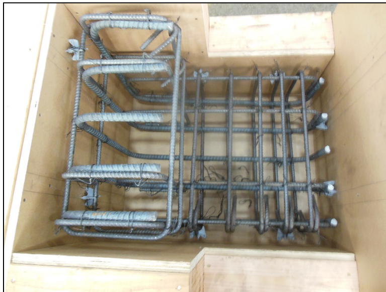
Figure 3.20: Cage for a specimen containing #4 (#13M) reinforcing bars across the interface inserted into constructed formwork
