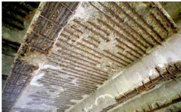
Figure 1.1: Accumulation of corrosion products at the surface of the reinforcing steel have caused the concrete to spall, exposing the reinforcing steel to further corrosion. This picture was taken at Big Creek Bridge prior to restoration ( Covino, et al. 2002 ).
