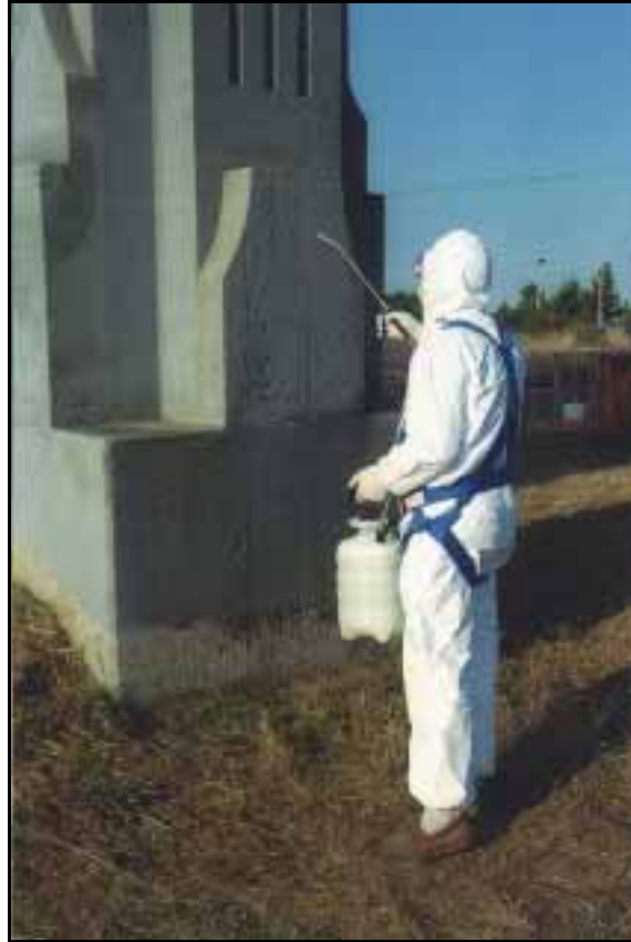
Figure 4.6: Application of humectants to the base of a bent on the Yaquina Bay Bridge
