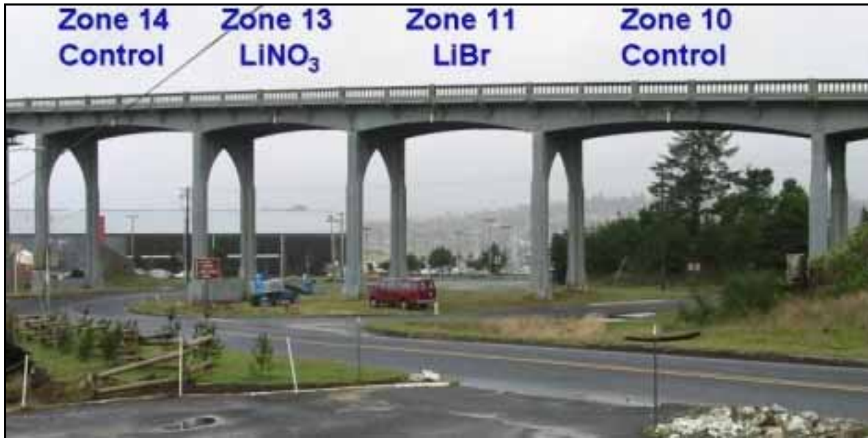
Figure 4.4: The four field test zones on the Yaquina Bay Bridge. Each zone includes column and soffit areas. Zone 14 is closest to Yaquina Bay. The closer a zone is to the ocean, the higher the expected \text{Cl}^- level and the lower the expected circuit resistance.
