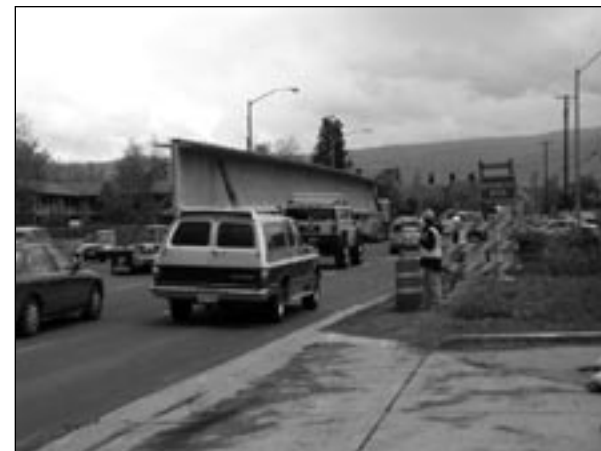
165-foot steel reinforced concrete beams are moved into place on the South Medford Interchange project.
