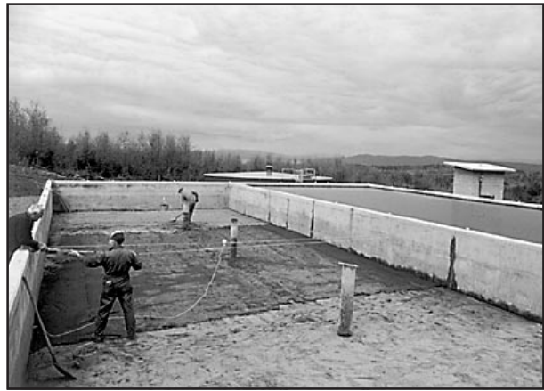
Photo 8-2. Slow sand filter, with schmutzdecke being scraped.
