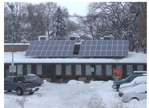
Solar array on the Pendleton State Office Building in December 2008
