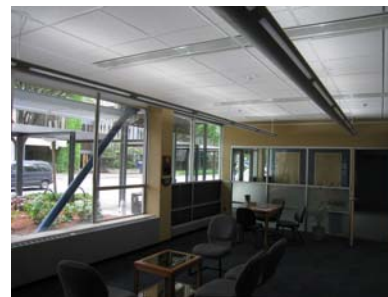
Chilled beams and indirect lighting highlight the innovative energy conservation measures incorporated into the Eugene State Office Building
