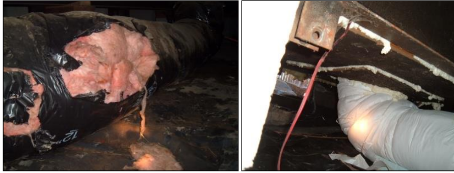
Damaged Flex Duct
