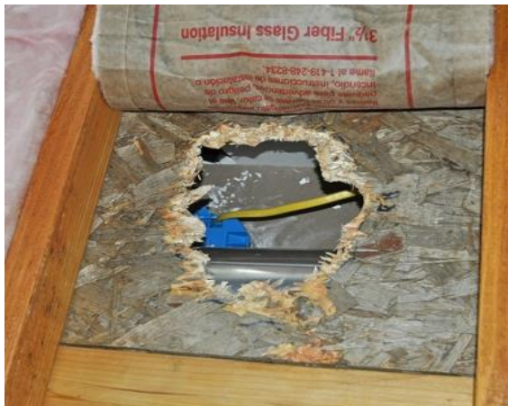
Prepare work area by removing existing insulation and debris from top ceiling
