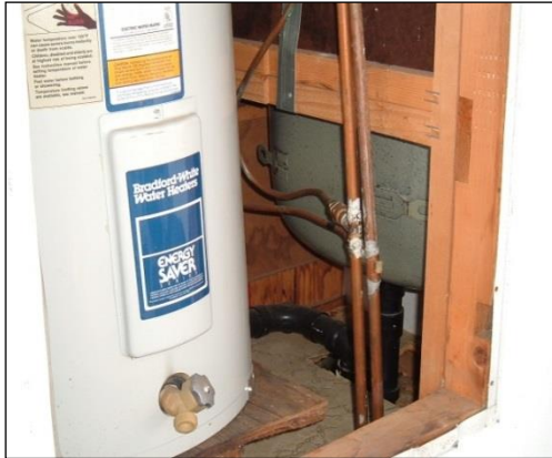
Water heater/bathtub penetration
