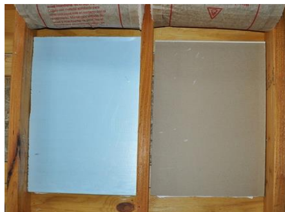
Step 2: Cover openings with rigid material. XPS or sheetrock may be used. Secure in place using screws.
