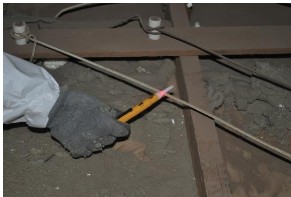
Non-Contact Testing of K&T Wiring
