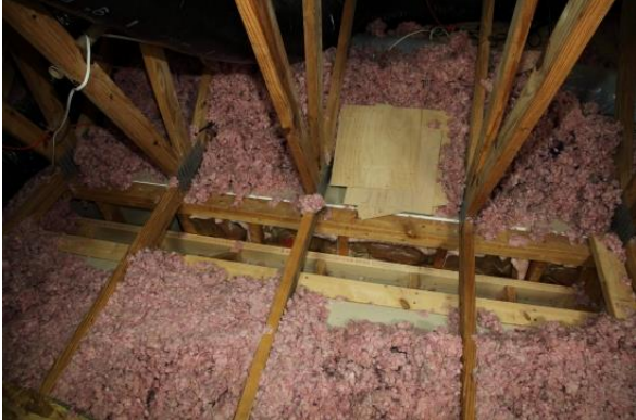
Seal top of soffit: Before- Wall cavities are open to the attic allowing for air leakage into the attic.
