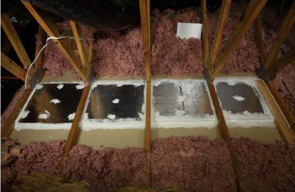
After: Top of soffit capped with rigid material, secured and thoroughly sealed.
