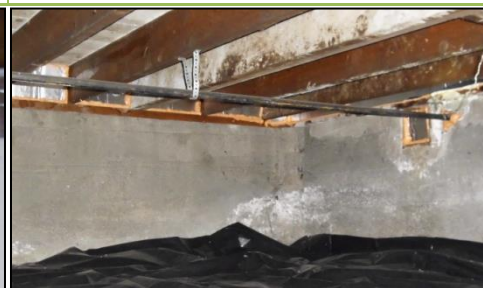
Rim joist insulation & ground cover
