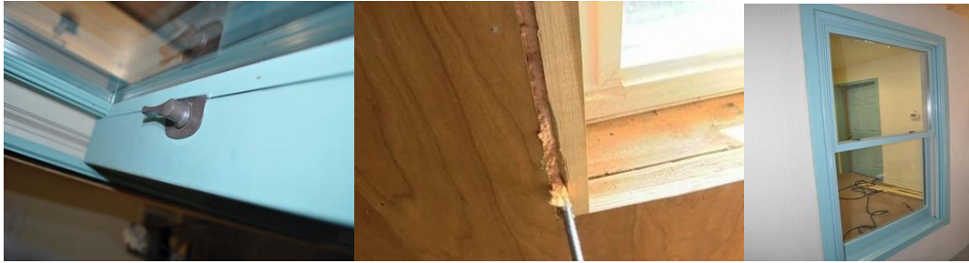
Verify window hardware works properly Foam or caulk gaps around the frame. Replace exterior trim and patch siding as needed
