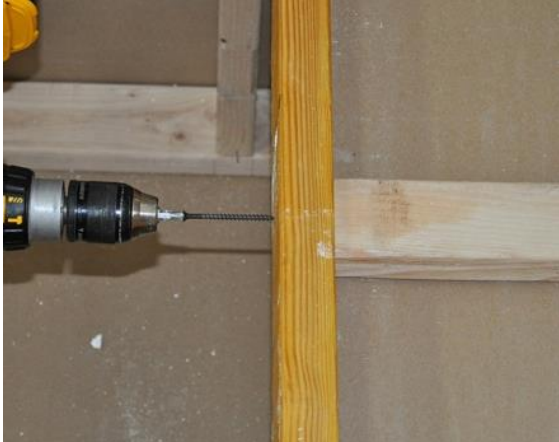
Ensure new bracing is secure by using screws or nails to fasten to the joist
