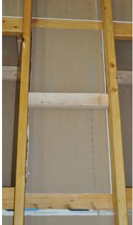
Once the chase is capped, the joint along the framed must be sealed
