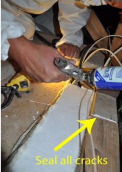
Sealant is used to fill in all cracks and gaps along edges of the cap
