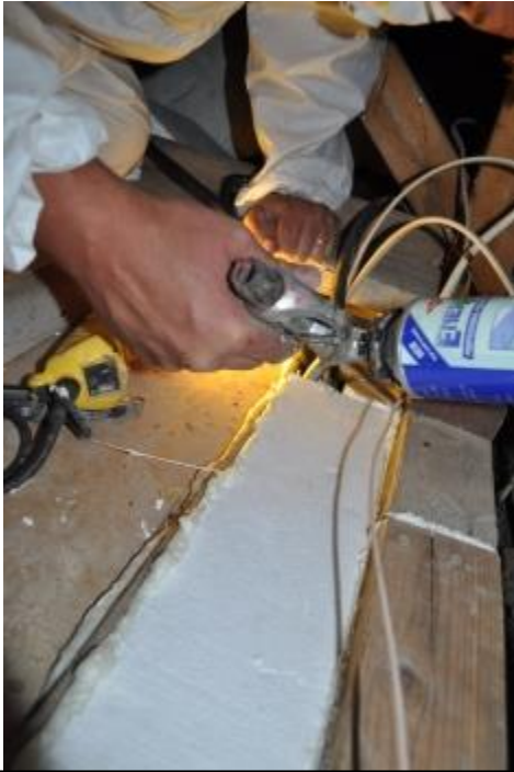
Sealant must be used to fill in all cracks and gaps along the edges of the chase cap
