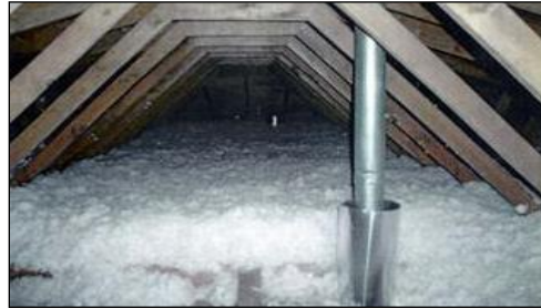
Shielded B Vent in Attic
