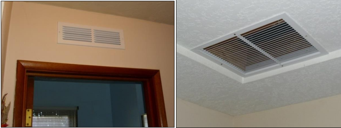
Through the wall bypass grille
