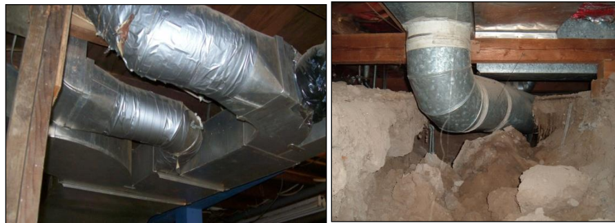
Before Mastic Sealing
