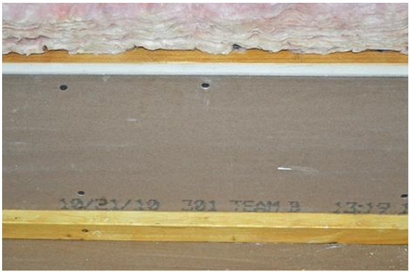
Option 3: Stud bay will be covered with rigid material, fastened and sealed.
