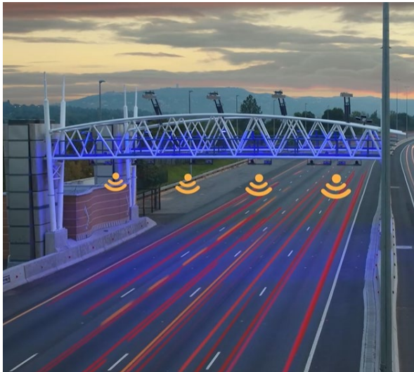
Figure 1-2. Electronic Toll Collection System
