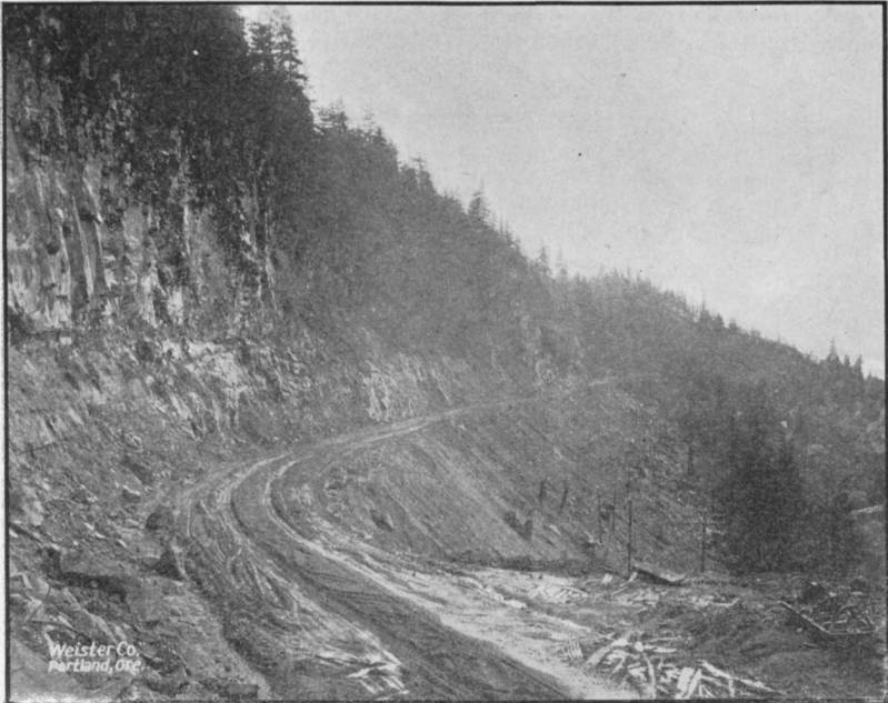
HEAVY GRADING ON RUTHTON HILL IN HOOD RIVER COUNTY. CONSTRUCTED IN 1917 AND 1918
